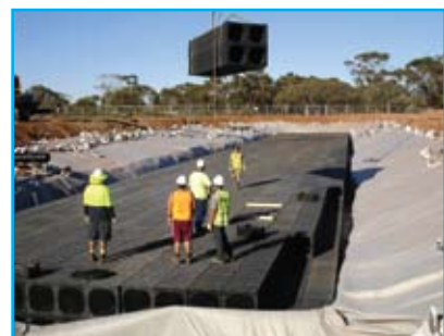
NSW (Council retention 850kL)
